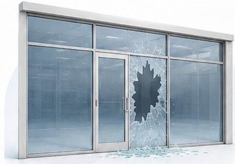
Broken Storefront Glass
